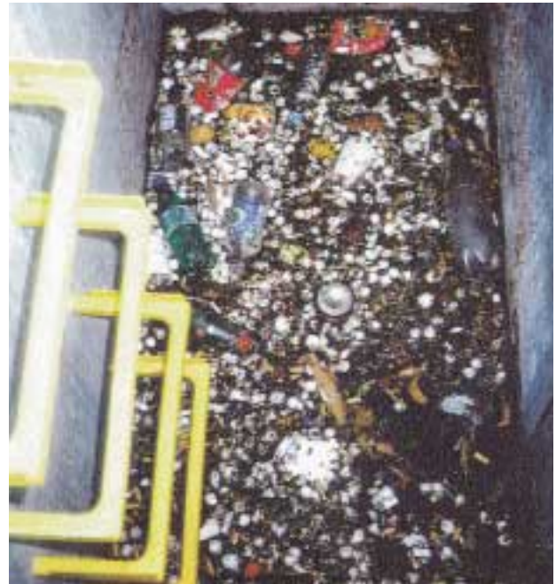
Gross pollutions retained in a Humegard™ storage chamber prior to cleanout.
